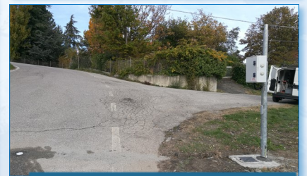
Road surface condition sensor – typical application
