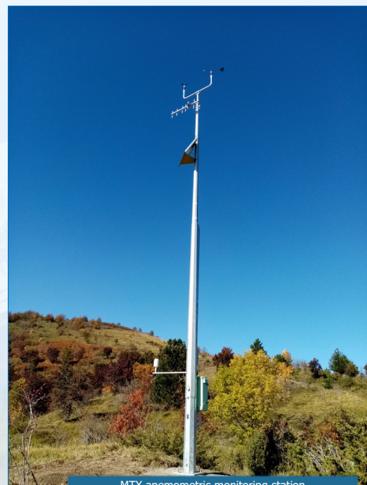
MTX anemometric monitoring station
